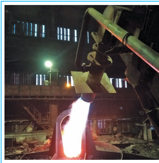
GNB-1500 high-speed burner in operating condition before immersion into a 250-ton ladle
