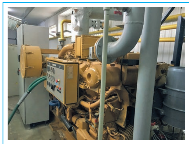
Generation equipment (electricity output is 500 kW)
